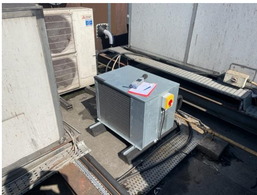
Figure 1 showing new ABS cooler
