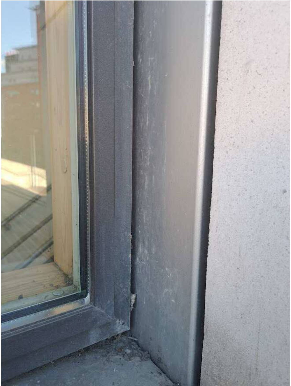
Fig 5: Existing stainless steel reveal flashing to be copied around new door reveal
