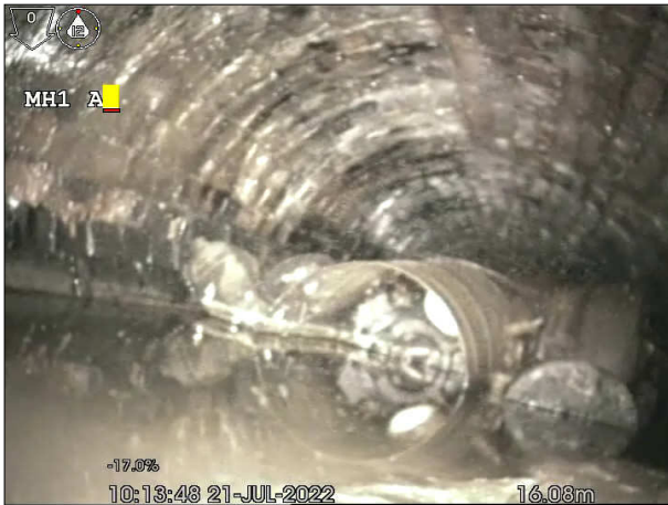
Photo: 14_14a, 00:00:00 18.1m, Debris, 95 % cross-sectional area loss
