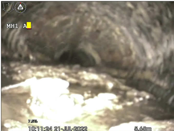
Photo: 1_8a, 00:00:00 6m, Debris silt, 45 % cross-sectional area loss, Changed
