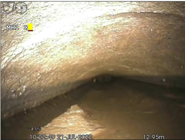
Photo: 27_11a, 00:00:00 12.95m, Survey abandoned, Remark: Unable to survey beyond blockage.
