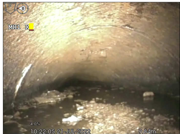
Photo: 25_9a, 00:00:00 9.84m, Debris silt, 40 % cross-sectional area loss
