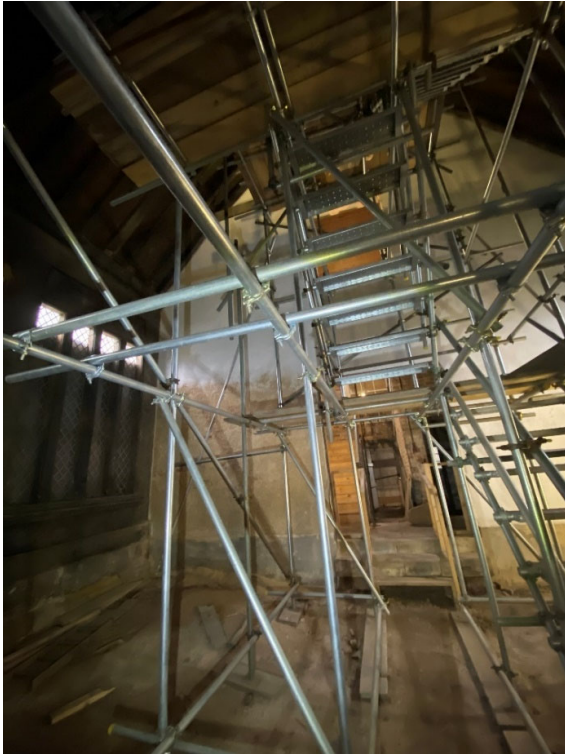
Figure 1 Area of defective plaster
