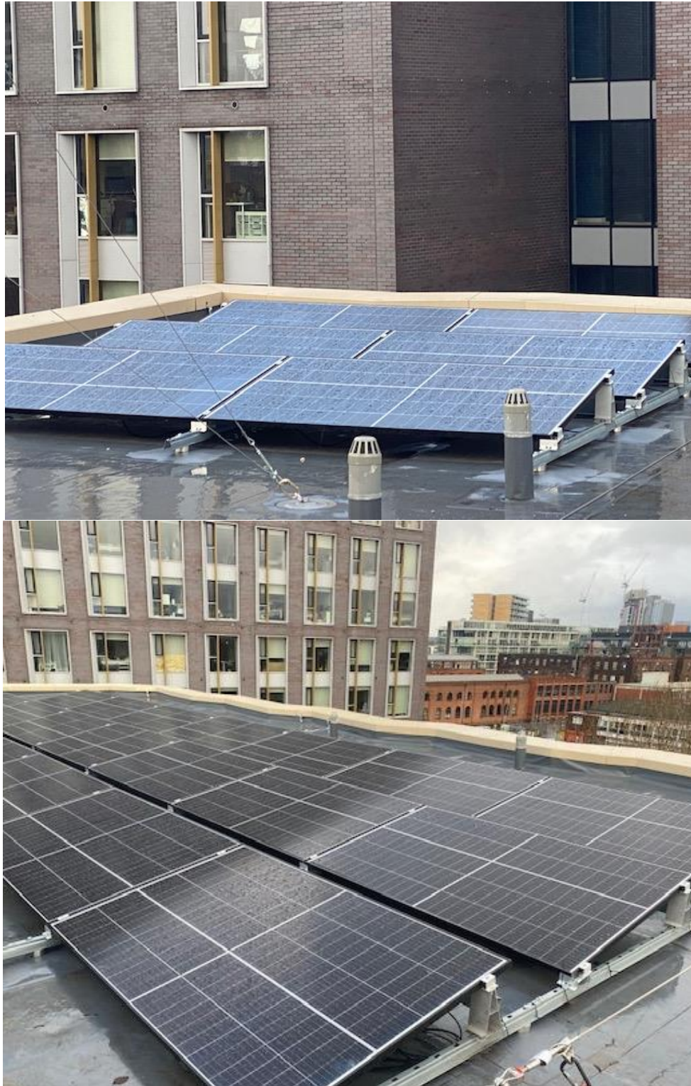
Fig 8: PV Panels to Roof
