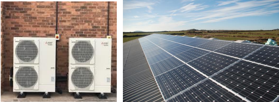
Figure 3 – ASHP and PV panels
