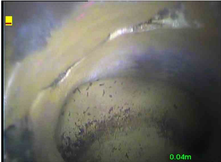
, 00:00:11, 0.40 m Crack, circumferential from 9 o'clock to 3 o'clock
