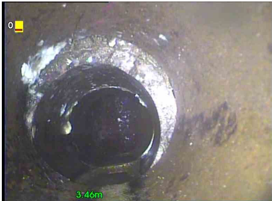
, 00:01:17, 3.46 m Joint displaced, medium
