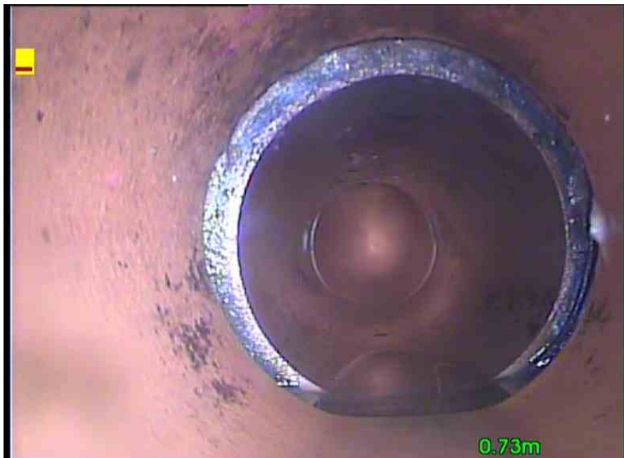
, 00:00:14, 0.73 m Joint displaced, medium
