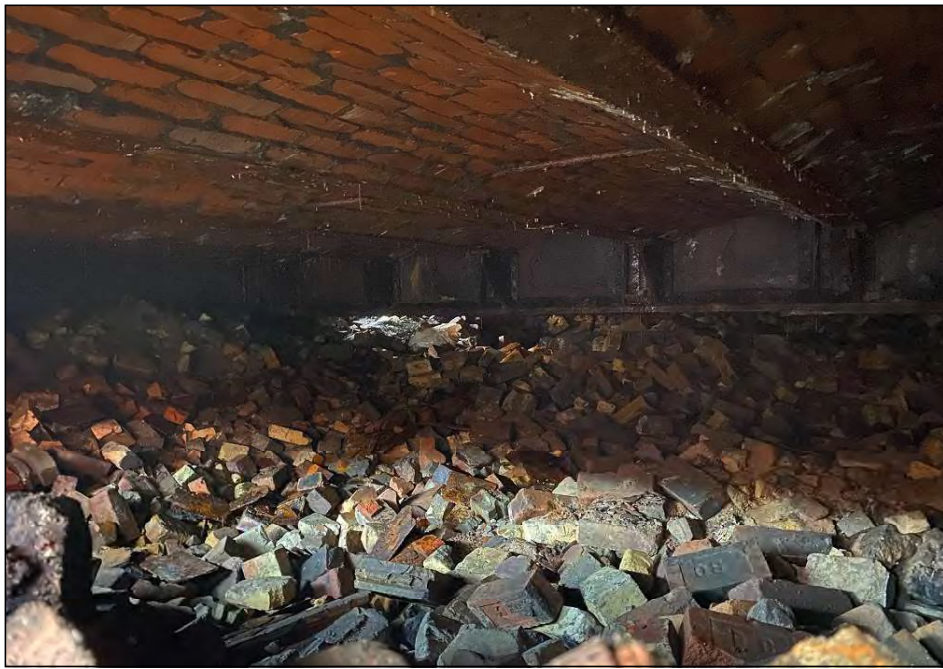
Plate 24. Open void beneath beam, looking northeast
