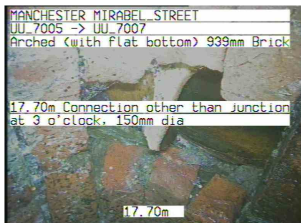
UU_7005X_4716ee5e-008a-40ef-99b1-78fa0c5b3197_20220914_101024_287.jpg, 00:03:03, 17.70 m Connection other than junction at 3 o'clock, 150mm dia
