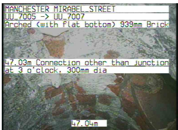
UU_7005X_37ba41dc-8feb-4ca2-810f-908c66b61ced_20220914_103110_290.jpg, 00:07:25, 47.03 m Connection other than junction at 3 o'clock, 300mm dia
