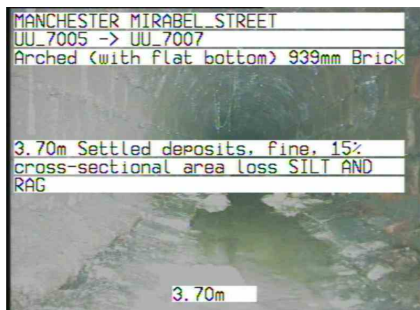
UU_7005X_5a572f83-b0e1-4d16-8fd0-bffd17460e10_20220914_100801_731.jpg, 00:00:56, 3.70 m Settled deposits, fine, 15% cross-sectional area loss, SILT AND RAG
