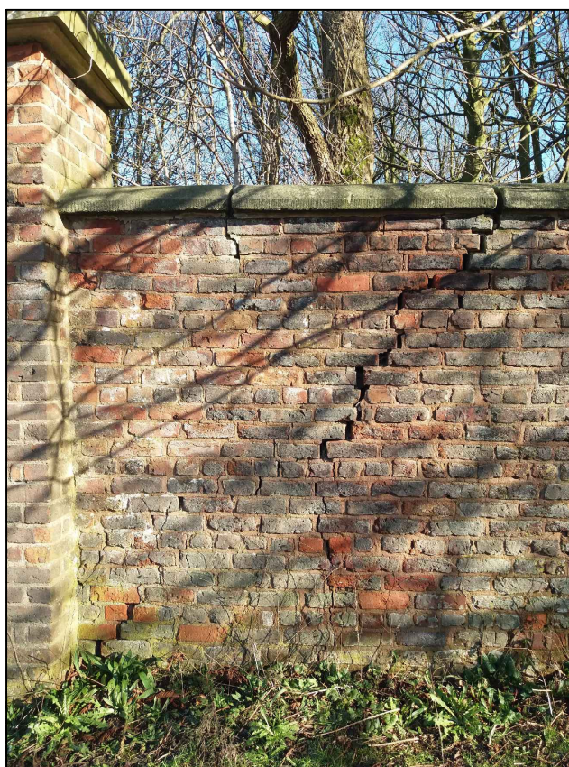
Photo 3: Stepped cracking to brickwork.
