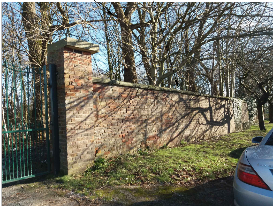
Photo 2: General view of damaged section to right hand side of pier.
