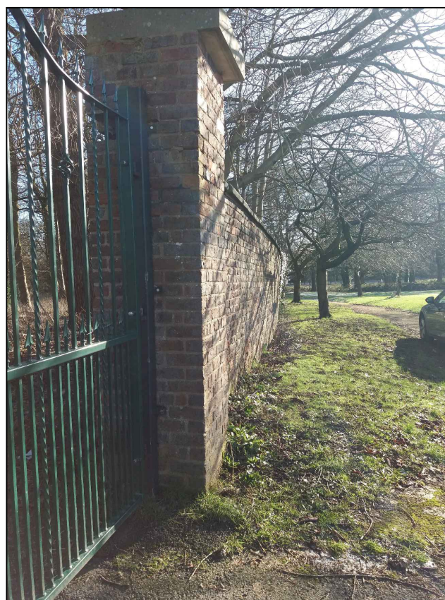
Photo 4: Outward lean to wall.
