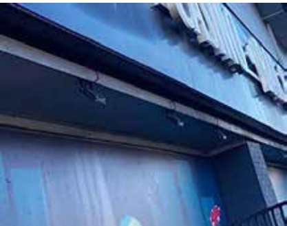
Existing illumination ITEMS 05 & 06
