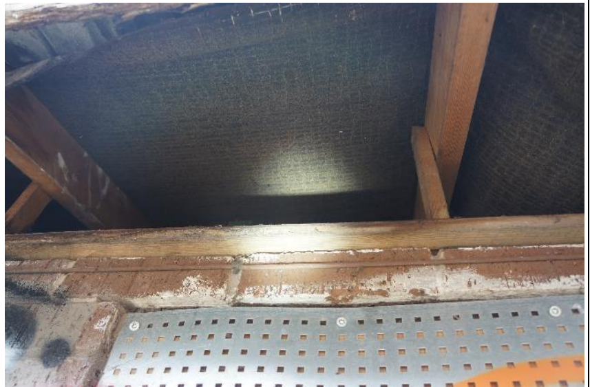
Figure 13: Large section of missing soffit on the single storey extension leaving a gaps allowing bats or birds to enter the building.
