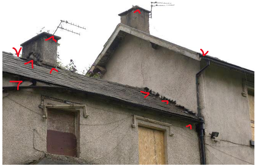
Figure 14: North elevation, showing missing lead and mortar with some gaps in roofing materials marked in red.
