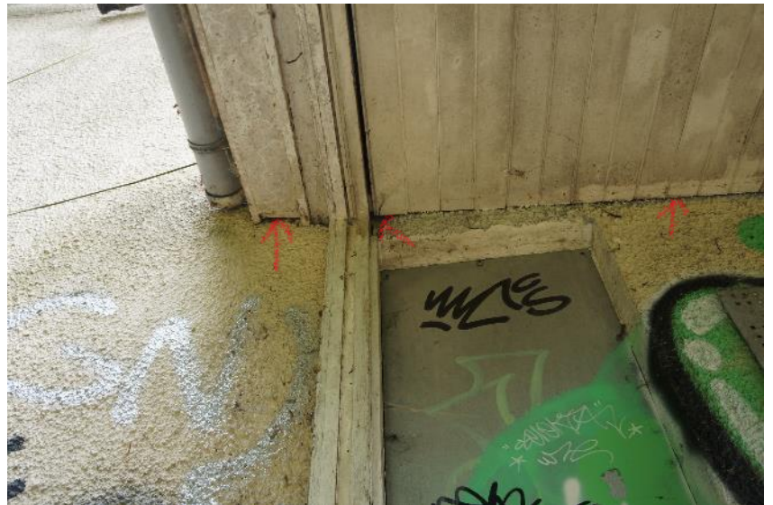
Figure 15: Gaps to the wall on the underside of the north elevation porch cladding.
