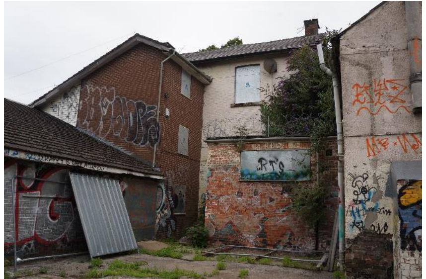
Figure 10: South elevation showing shrubs growing from the extension roof.
