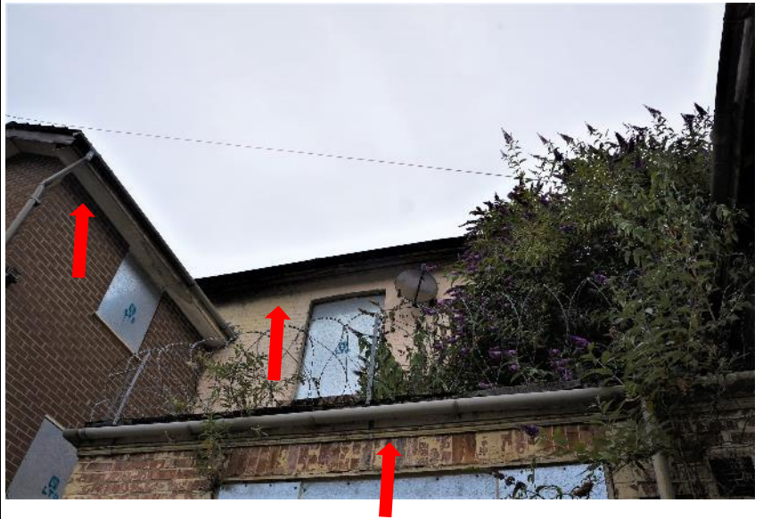
Figure 12: South elevation showing examples of gaps in timber roofline materials..
