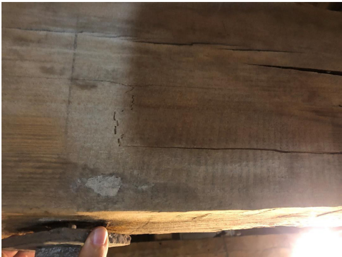
Close up of roof truss cracking, to the south of propped trusses in Bay 2, with cracking of main tie.
