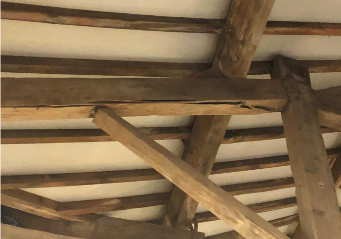
Roof truss in Bay 1 showing high level splitting in principal rafter.
