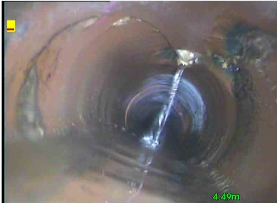
, 00:00:50, 4.49 m Crack, circumferential from 8 o'clock to 3 o'clock
