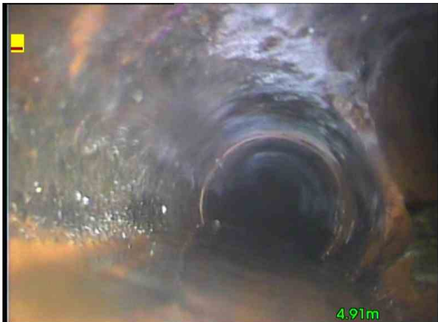
, 00:01:10, 6.49 m Crack, circumferential from 12 o'clock to 4 o'clock
