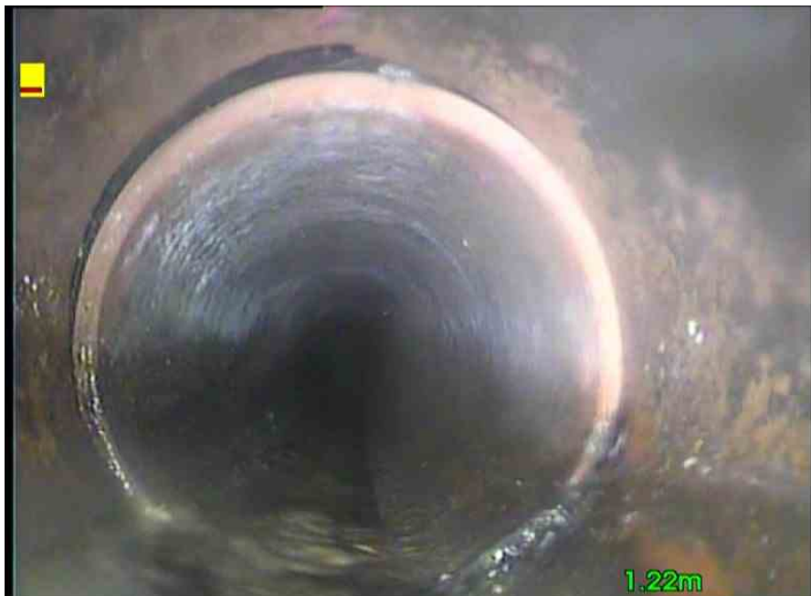
, 00:00:25, 1.22 m Broken pipe at joint from 9 o'clock to 1 o'clock ,
