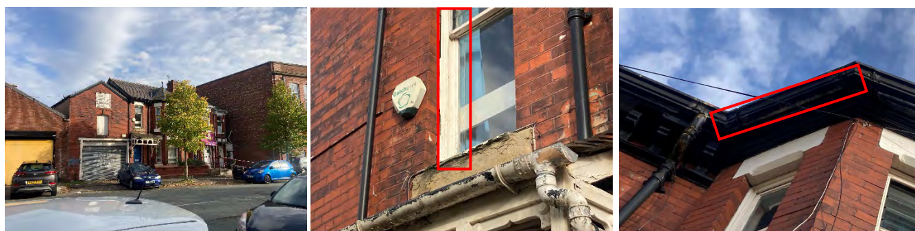
Photograph 7: a) Western aspect of Building 4. b) Crevice between window frame and brick c) Crevice within soffit.
