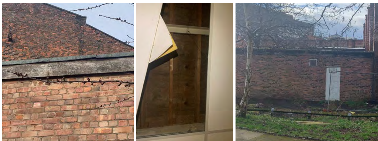
Photograph 11: a) Lifted bitumen along wooden bargeboard, eastern aspect of B07. b) wooden boarding, above dropped ceiling, c) building eastern aspect
