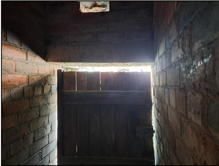
Photograph 2 showing gaps around the door in Building 1
