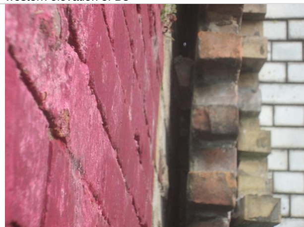
Photo 17: Gaps between brick layers at western elevation of B3
