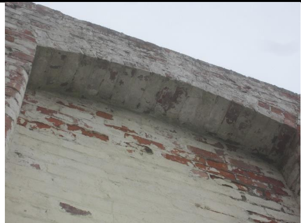
Photo 26: no gaps at bricked up window apertures / underrach at B4
