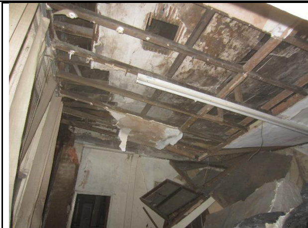
Photo 7: Damage of ceiling at first floor of B1
