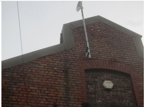
Photo 24: Gaps behind overlapping sheet cover at eastern elevation of B4
