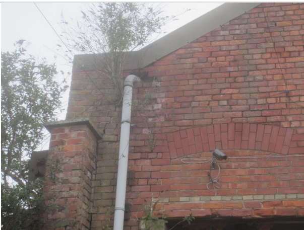
Photo 23: Cracks and gaps in brickwork at eastern elevation of B4
