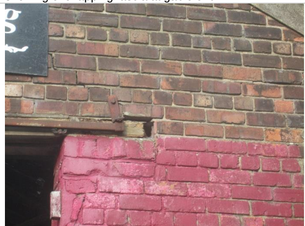
Photo 16: Holes in brickwork at B3 (western elevation)
