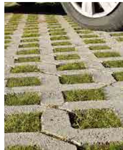
OVERFLOW CARPARK - TOBERMORE TURFSTONE GRASS PAVING SYSTEM
