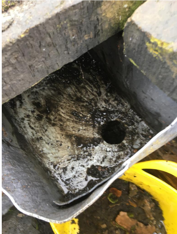
Hopper cleared of debris.
