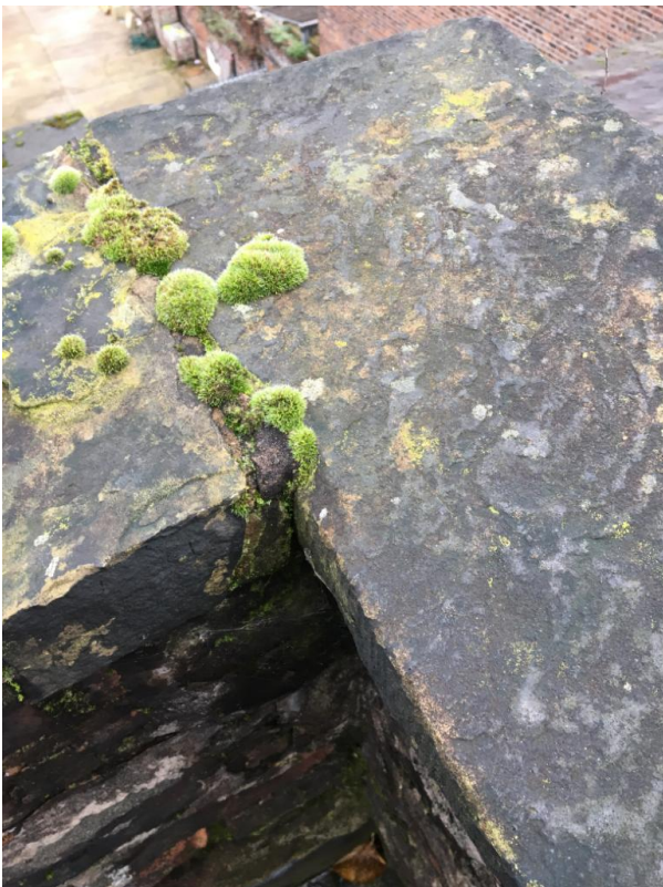
Failed coping stone mortar joint.
