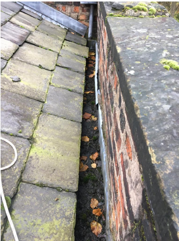
Gutter found full of debris.
