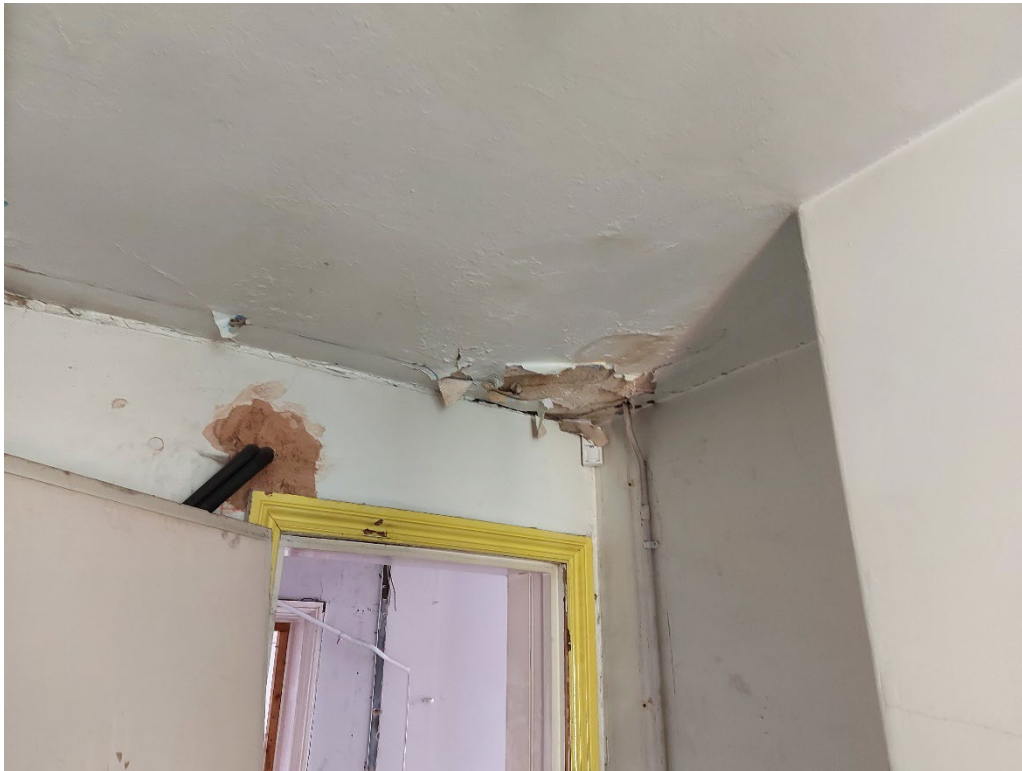
Photograph 7 Rear annexe, over entrance door – evidence of past leakage in lean-to roof
