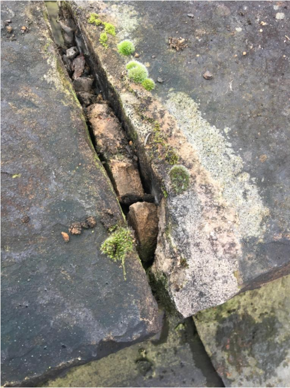
Failed coping stone mortar joint.
