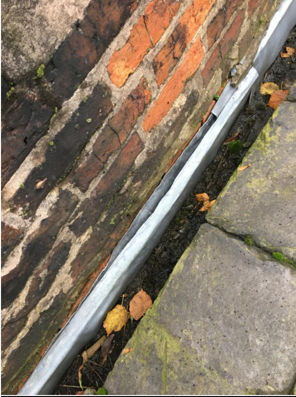
Gutter found full of debris.
