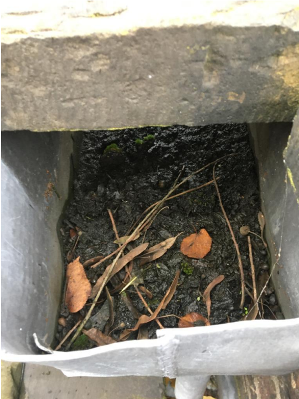
Hopper found full of debris.
