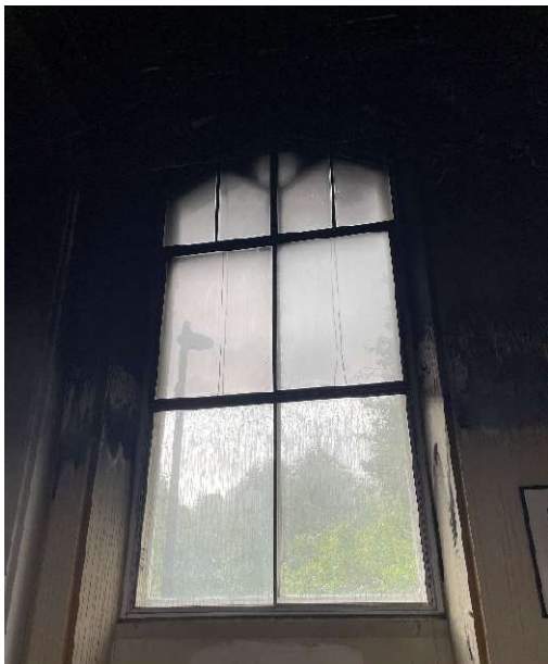
Whiteley Hall - Damage to Secondary Glazing
