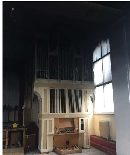
Whiteley Hall - Damage to Existing Organ
