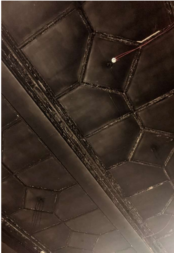
Whiteley Hall - Fire Damaged Ceiling
