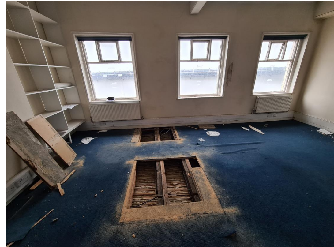
Figure 4: Second Floor front room looking towards front elevation with dishing in floor plate
