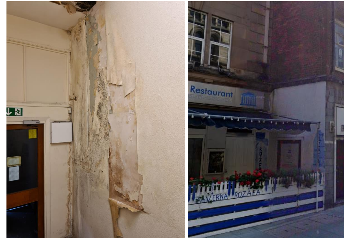
Figure 2: View of water damage to party wall and perished downpipe on adjacent property
