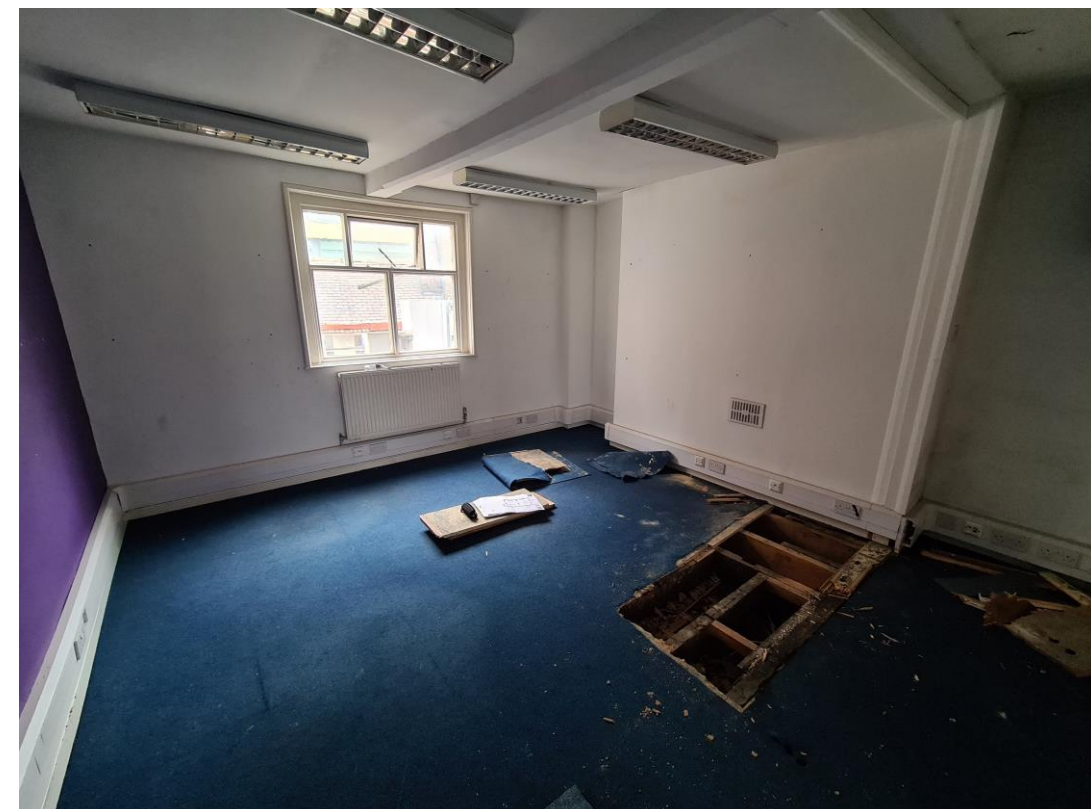
Figure 5: Second Floor rear room looking towards rear elevation with dishing in floor plate
