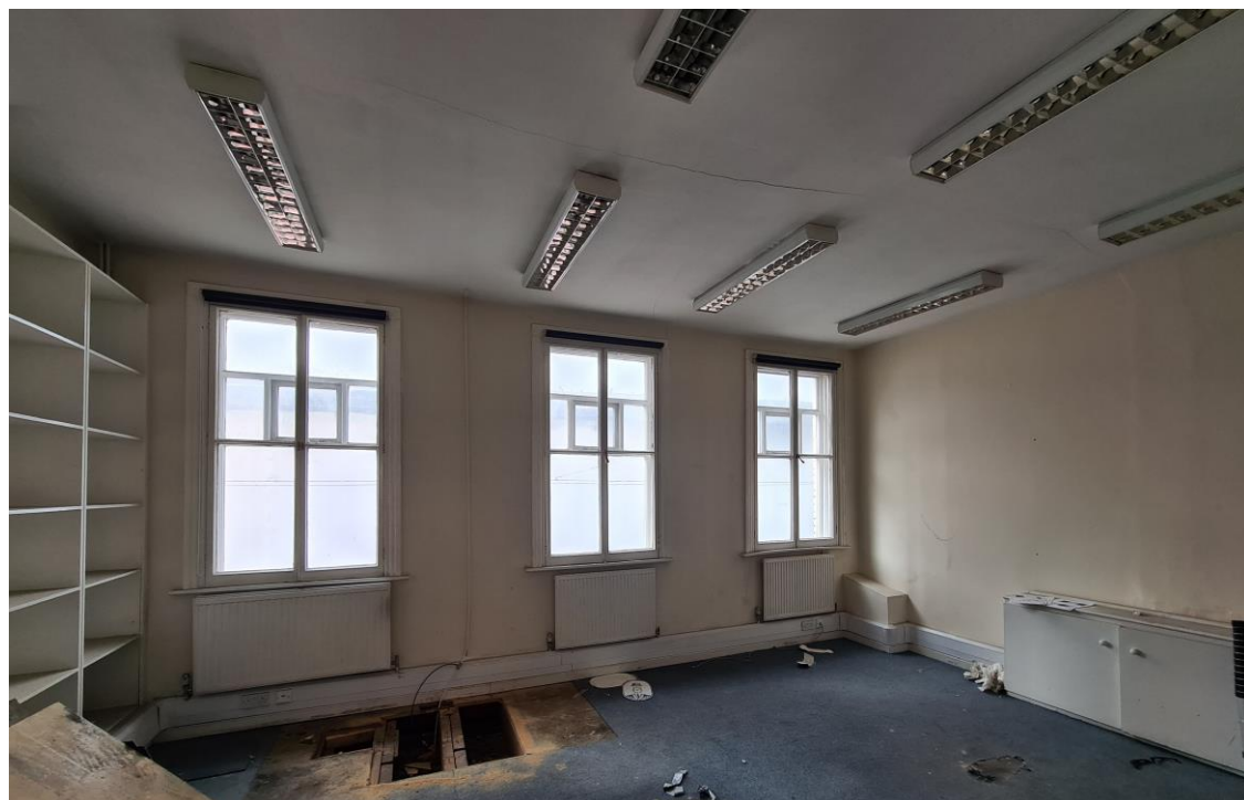
Figure 3: First Floor looking towards front elevation with cracking to ceiling
