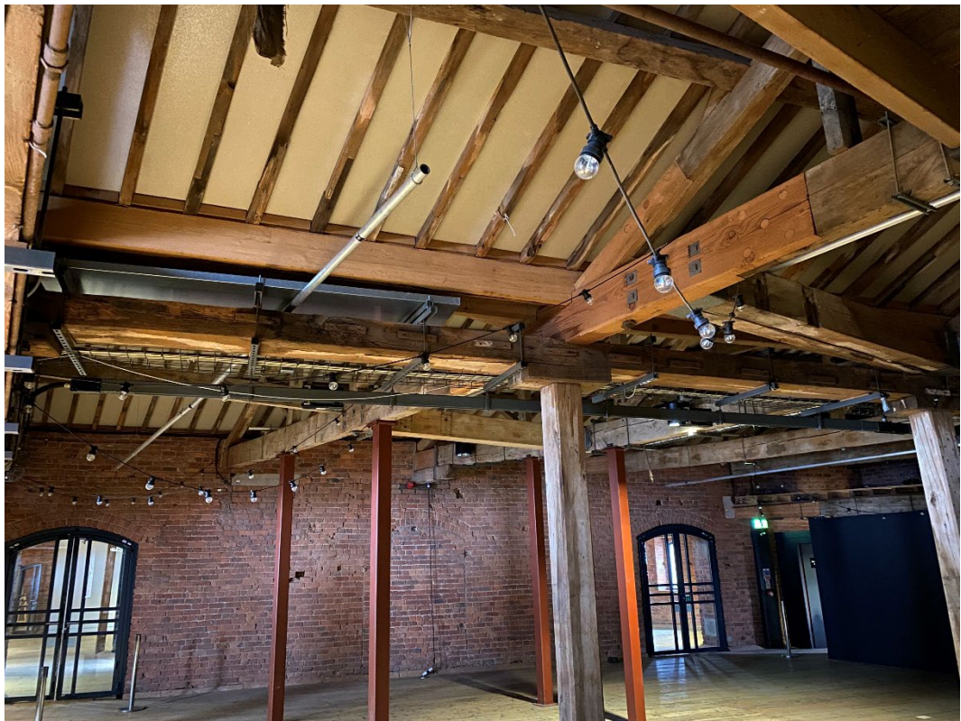
Figure 16: Later steel columns inserted beneath major truss within Bay 2 and intruding into the otherwise open space. Also note carefully spliced in timber repairs to the truss which are more sympathetic to heritage character while still being legibly as a repair.
