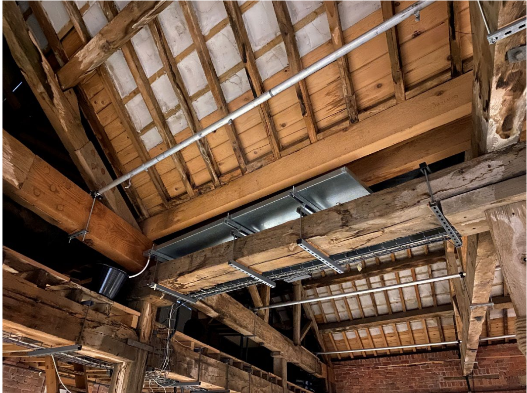
Figure 17: torching in Bay 4 with sarking boards indicating the different finish to accommodate and support the lead of the valley gutter. None of the actual roof surfaces or finishes are visible internally.
