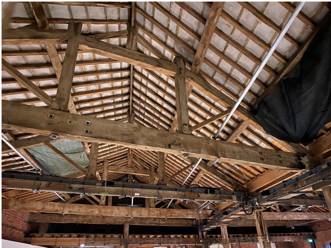
Figure 10: Bay 4 roof today, note netting in place to catch the falling torching
