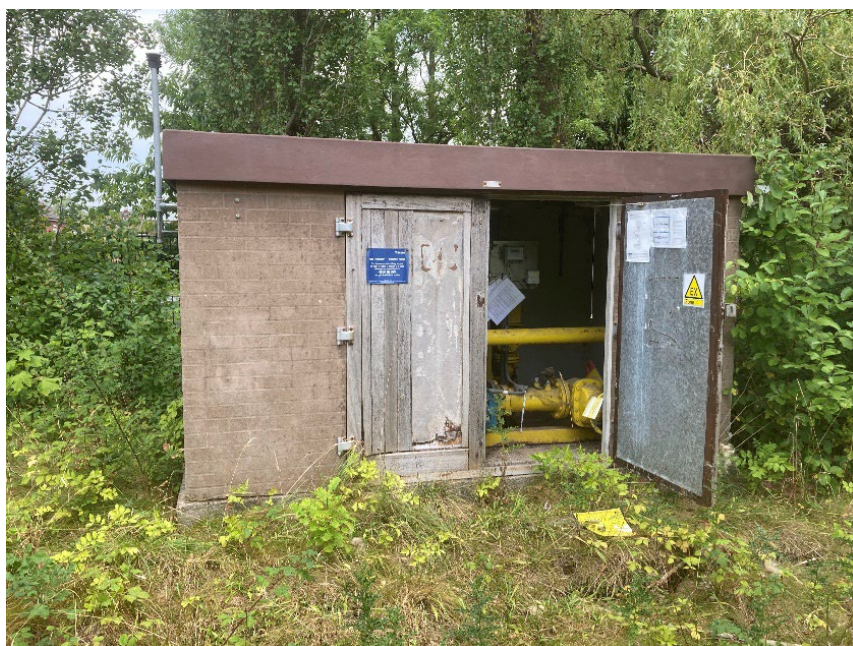
Photographs 2 - Building housing gas mains.
