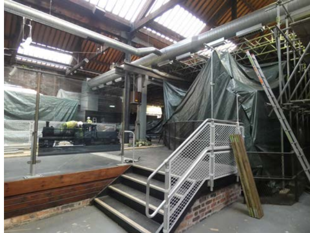
A.41 View of modern gantry and ductwork over the platform (Insall).
