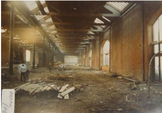
2.17 c.1981 View of the Power Hall (SIM Archive YA2007.4129. Licence CC-BY-NC-SA 4.0)
