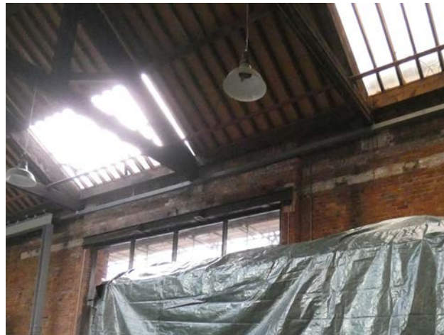
A.27 Traces of limewash on the south wall (Insall).
