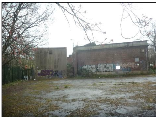
Photo 1: Vegetation colonising hard standing
