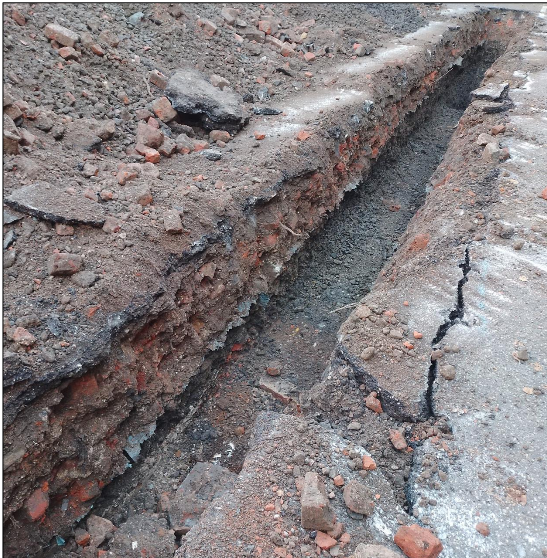
Plate 8: Trench 2 looking south, cracked and collapsing trench edge visible on right
