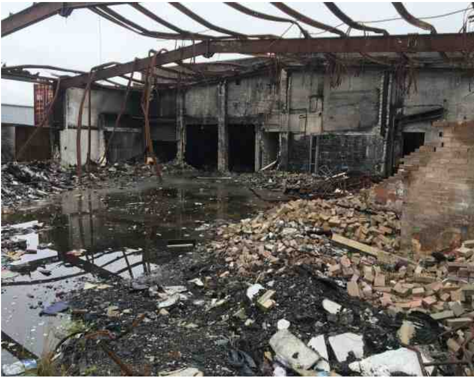
Photograph 5: View of the extensive fire damage to the current building, pooling surface water and rubble.
