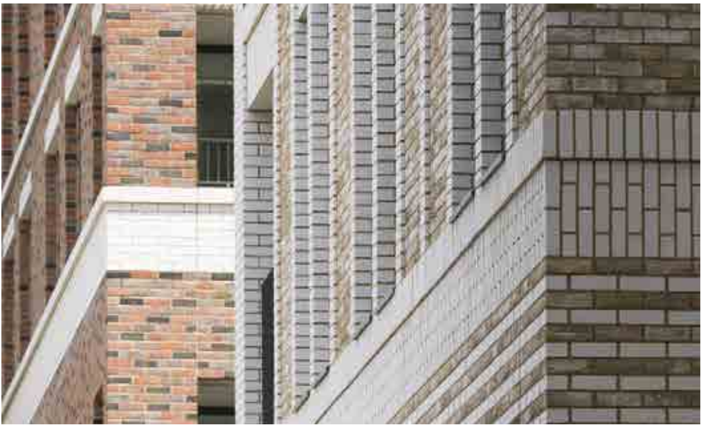
CONTRASTING BANDING AT LOWER LEVEL
