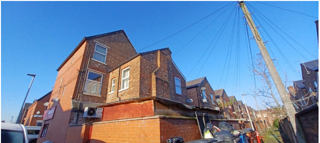
Figure 1. Rear view of the property, depicting the unauthorised structure and unauthorised air conditioning unit.
