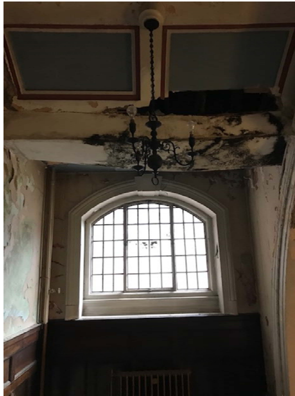
Soffit Collaspse around beam; dry rot
