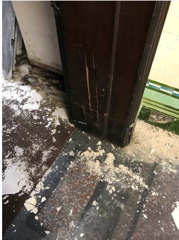
Dry rot decay to door jamb reveal
