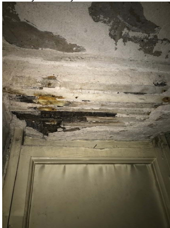
Dry rot decay to reveal soffit in WC
