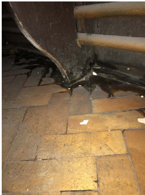
Visible wetting to Parquet in Courtroom
