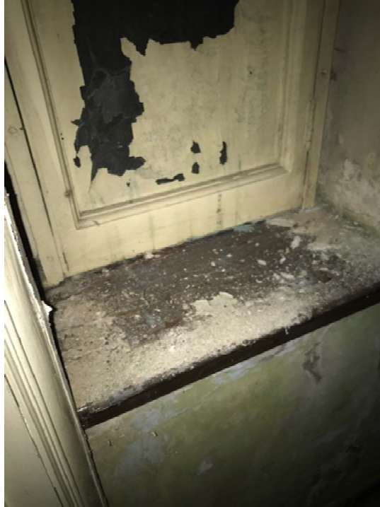
Dry rot decay to cill in WC
