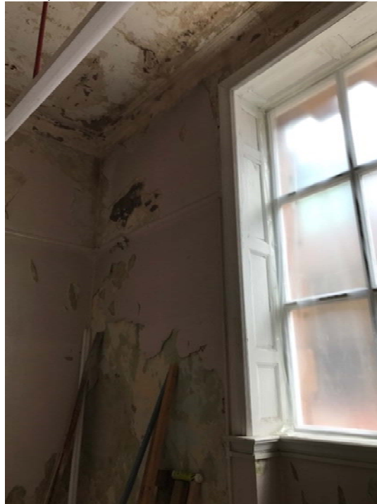
Residual dampness to wall and soffit around window reveals
