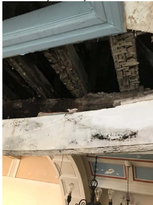
Dry rot decay to soffit
