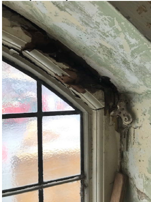
Dry rot decay to window Frame
