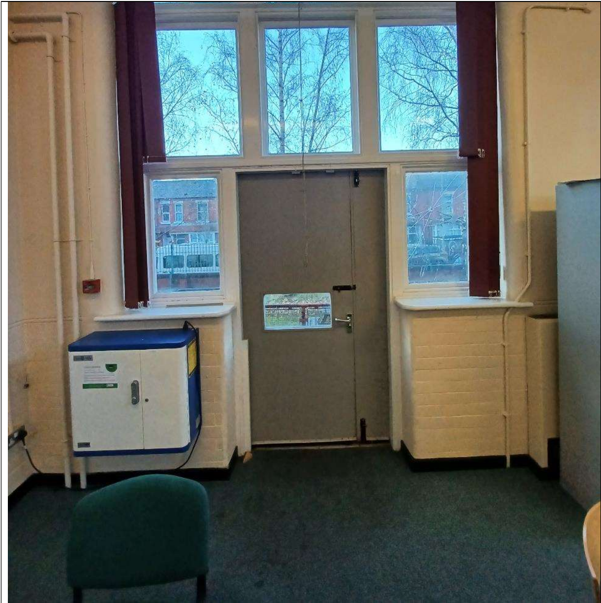
Photograph: 4 - Final exit door with no exit sign
