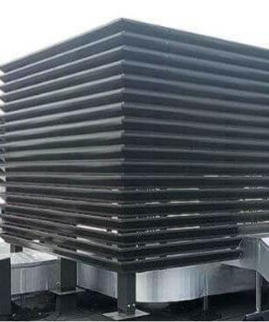
6 Plant Louvre Screen
