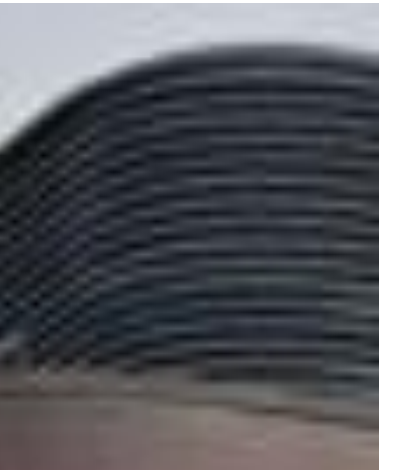
6 Oak Road Treatment Centre Plant Louvre Screen
