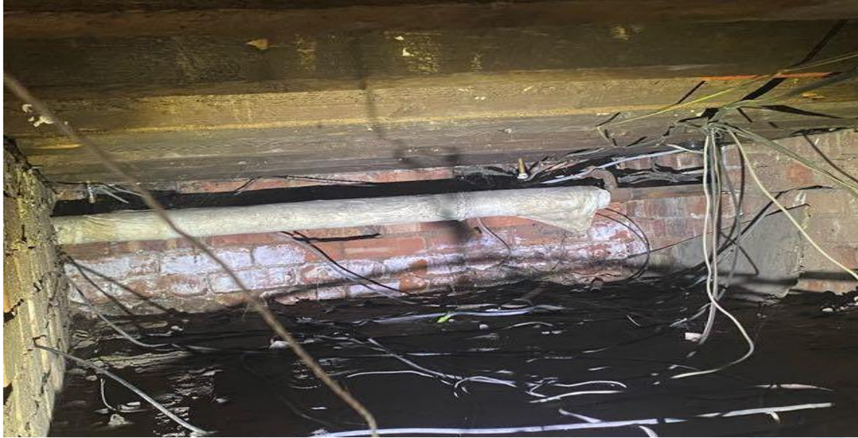
Pipe work to floor void
