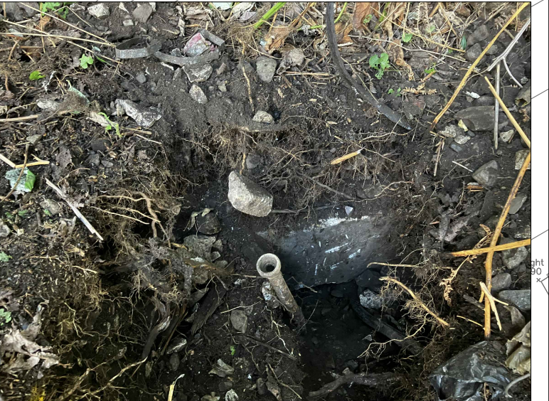
OLD PIPES ENCOUNTERED WITHIN PIT. UTILITY DUCT APPEARS TO CONTINUE IN E-W DIRECTION ALONG FENCELINE 0.40mbgl.
