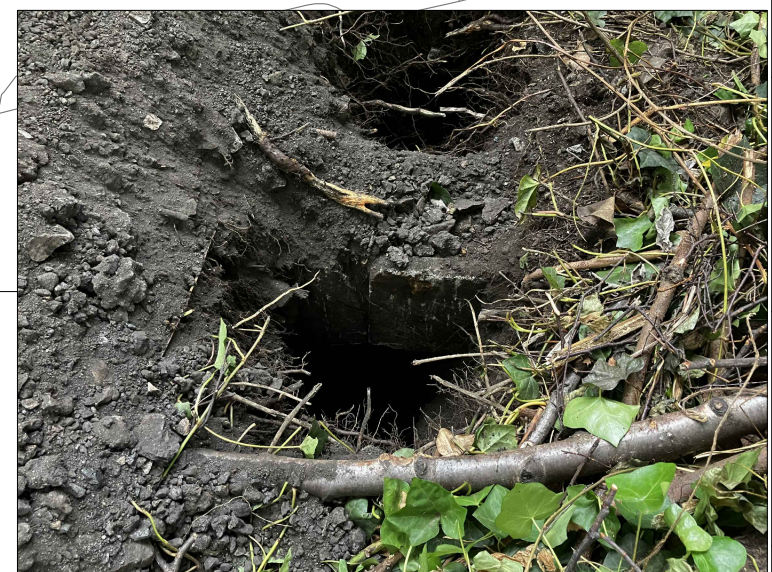
UTILITY DUCT ENCOUNTERED RUNNING E-W ALONG FENCELINE
