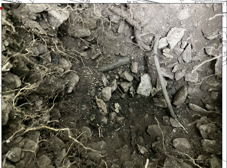
OLD CABLES WITHIN PIT @ 0.60-0.80mbgl.
