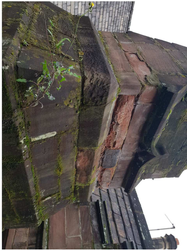
High level stone work to chimney - surface erosion to stonework
