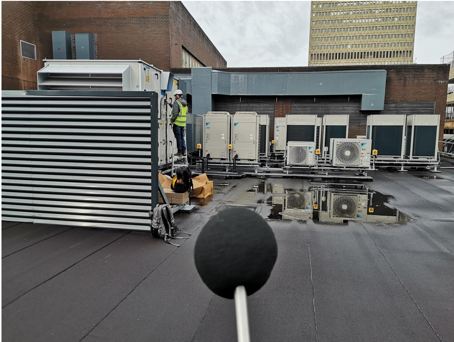
Figure 2:3 – Installed plant and measurement photograph
