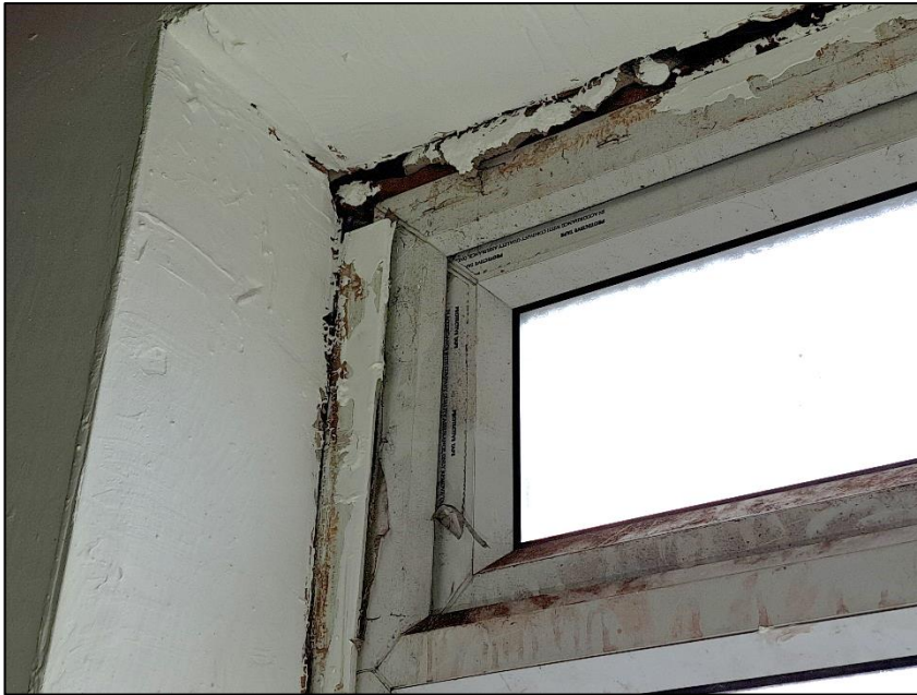
Photograph 9 showing damage above one of the windows
