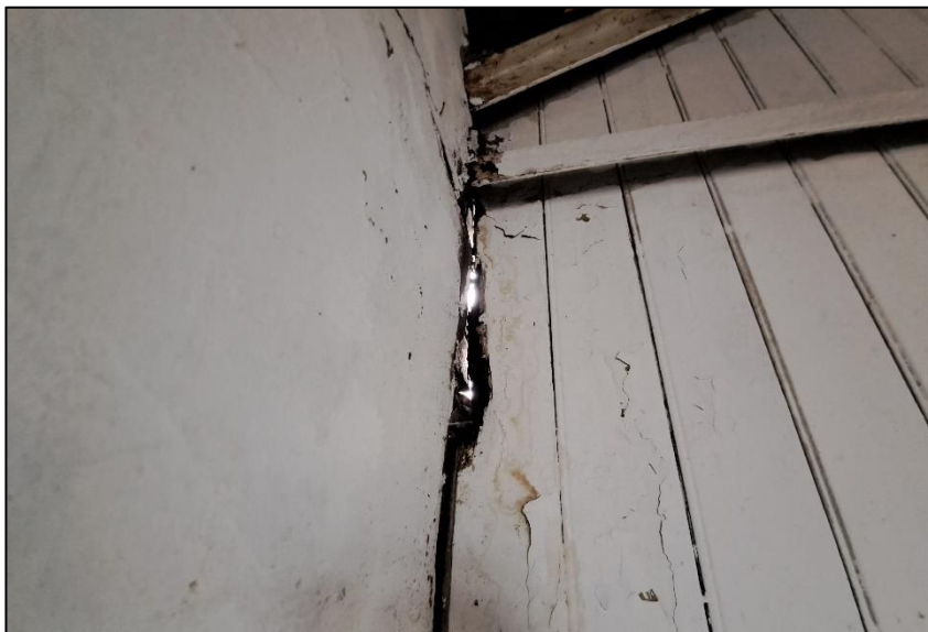
Photograph 8 showing one of the gaps in the corner of the uppermost floor
