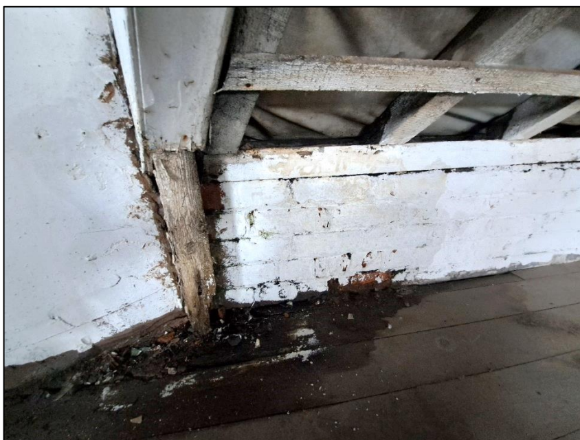
Photograph 5 showing an area of wood rot
