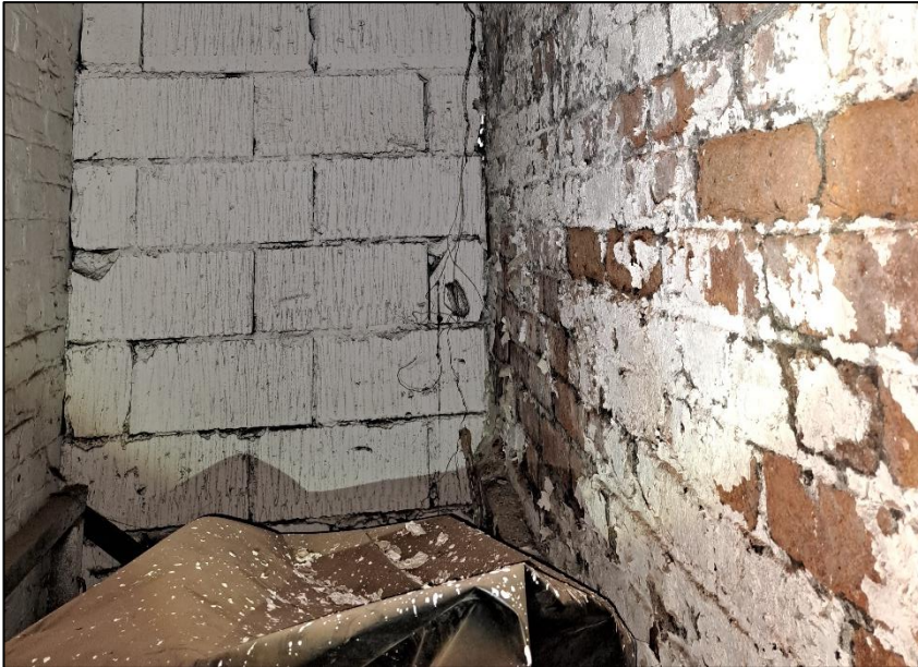
Photograph 7 showing the condition of the internal brickwork
