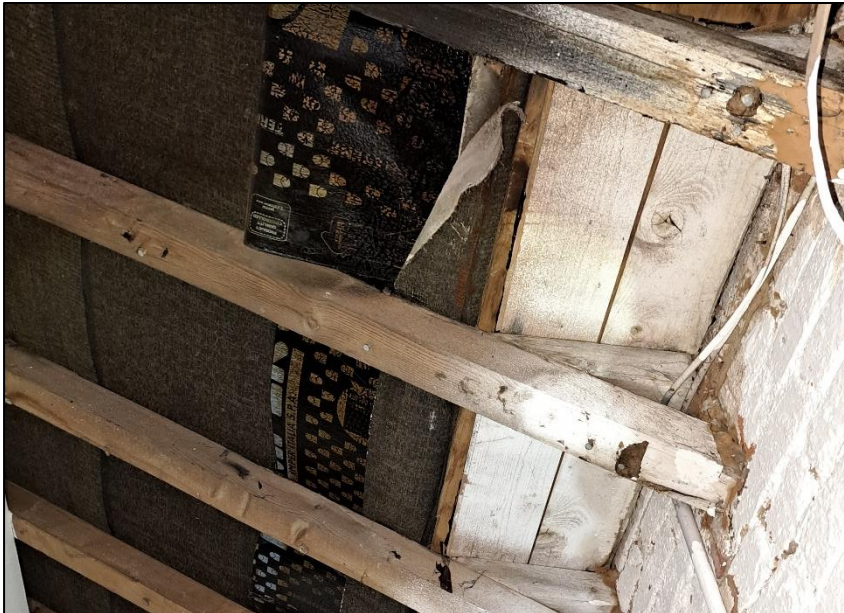
Photograph 6 showing an area of exposed roof lining
