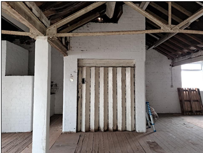
Photograph 10 showing the void and daylight above the lift shaft
