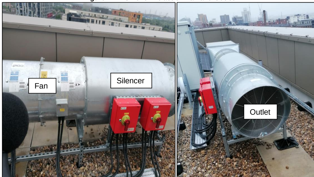
Figure 2.1 – Smoke Extraction Fan and Outlet
