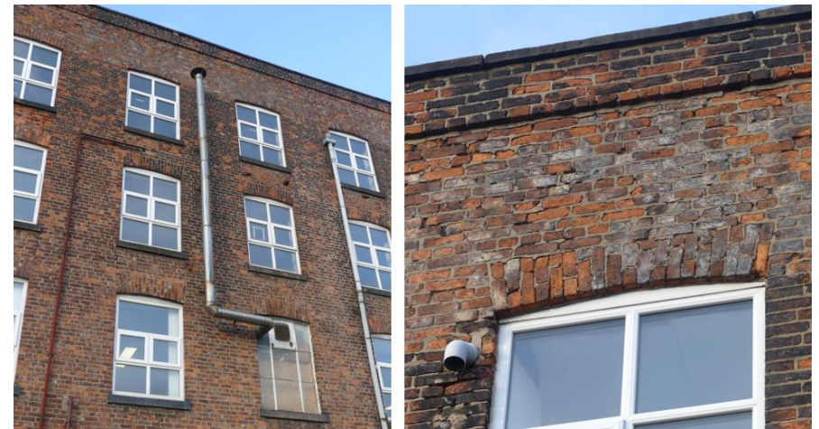
Figure 5.1: The existing uPVC windows, ventilation flue and defective brickwork below the parapet of the southern elevation
