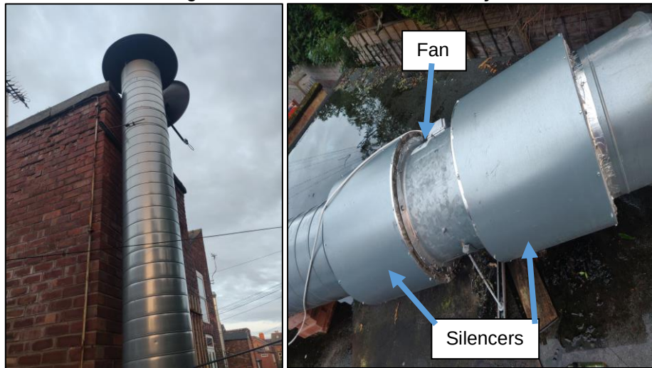
Figure 1.2 – Extractor Fan and Chimney
