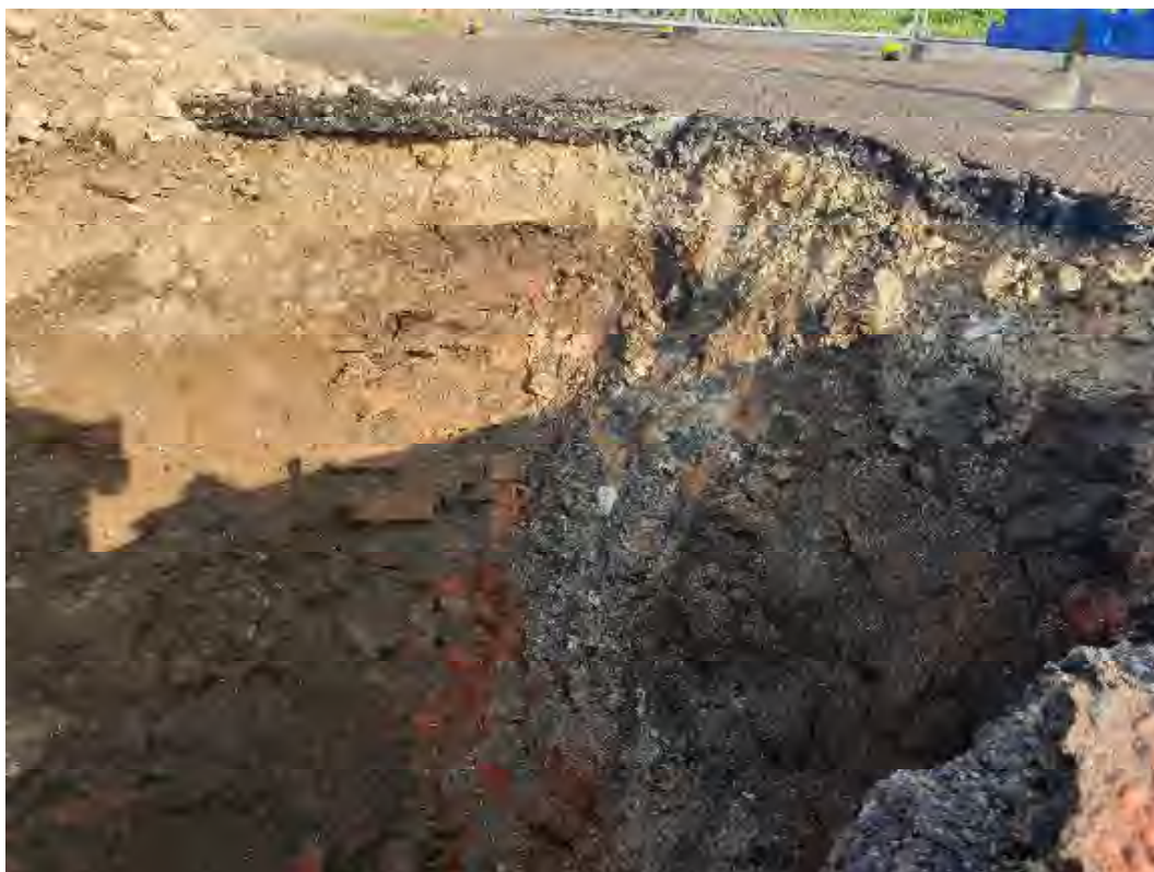
Photo No. 8: TPI04
