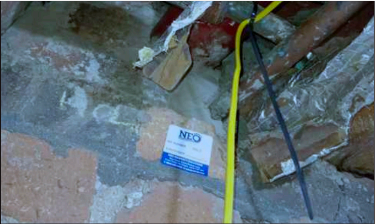
Images 15, 16, 17, showing examples of repair locations at PIN locations 0020:38, 60:38 and 53:38
