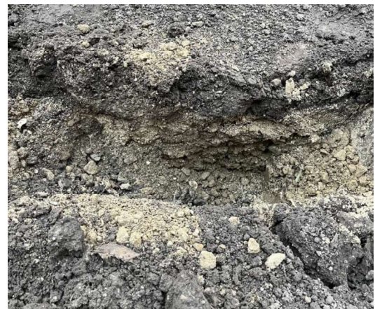
Photo 12: TP05 Close Up
