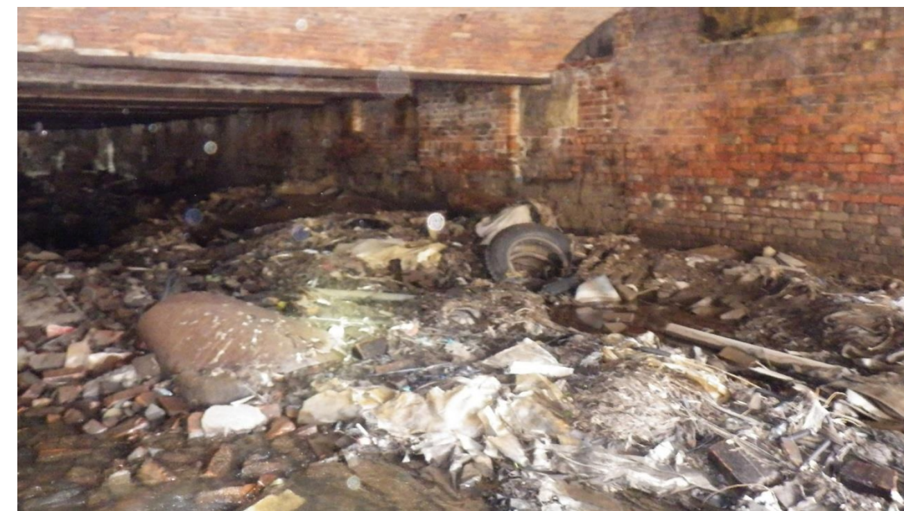
Figure 5-3 Debris build up within culvert
