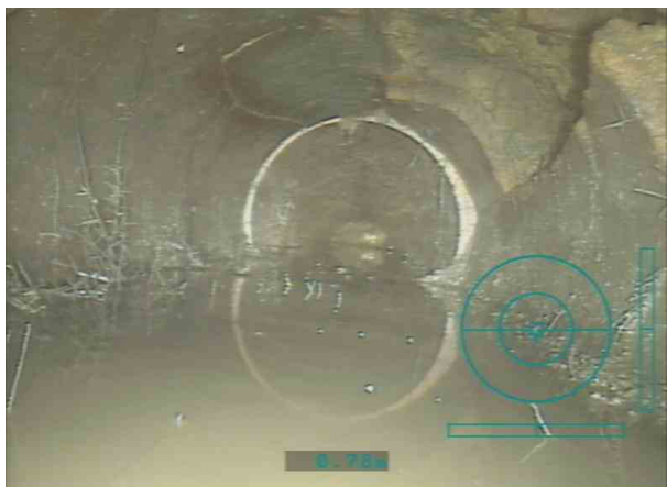
2202X_3c85dc51-271d-4ecb-8ab4-7ba6f2264d26_20191219_202629_924.jpg, 00:03:17, 0.78 m Survey abandoned, Due to amount of silt
