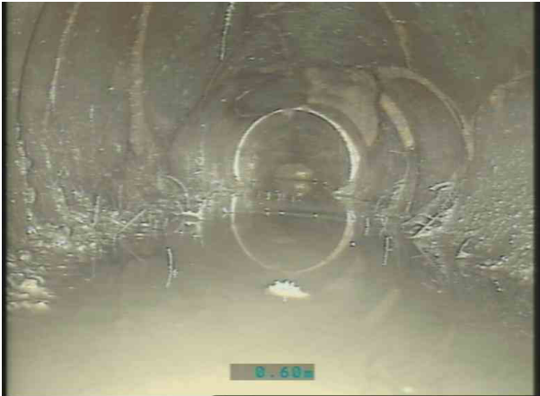
2202X_faa5824c-328f-4b59-8d4a-b95a0af8fc36_20191219_202346_967.jpg, 00:00:37, 0.60 m Fractures, multiple from 7 o'clock to 5 o'clock
