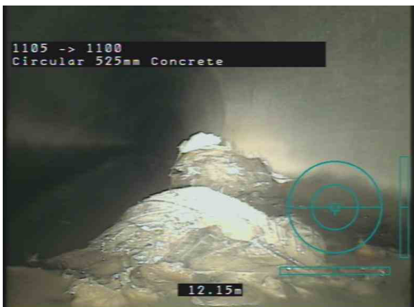
1105X_04d7ba1b-8c45-4777-839c-1492a72d1db0_20191218_213804_994.jpg, 00:09:04, 12.15 m Other obstacles, brick or masonry in invert from 4 o'clock to 7 o'clock, 20% cross-sectional area loss
