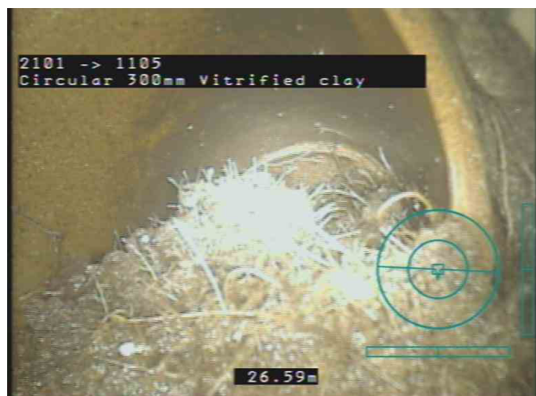
2101X_aff6f31d-438d-49fc-9cb5-d164974ebd40_20191218_24120_287.jpg, 00:10:39, 26.59 m Connection defective, connecting pipe is blocked at 10 o'clock, diameter: 150mm
