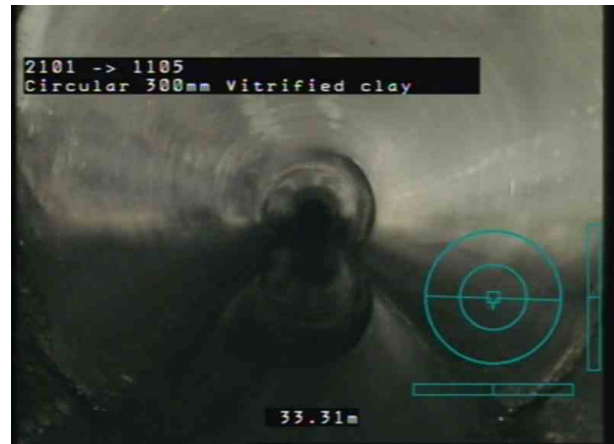
2101X_df33cf18-b4ab-4f51-898c-c87bf54343cf_20200109_082904_272.jpg, 00:15:31, 33.31 m Roots, fine at joint
