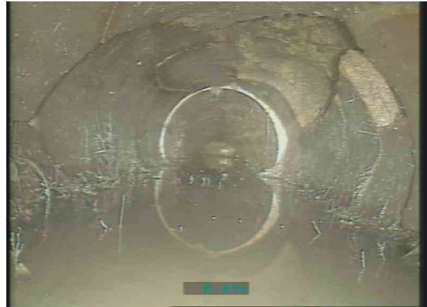
2202X_9e74917b-78b7-4495-8c04-d6319efe82de_20191219_202430_818.jpg, 00:01:18, 0.69 m Settled deposits, fine, 20% cross-sectional area loss
