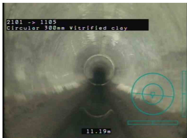
2101X_09cd2e99-ddea-4d5f-996f-3bdd47d71097_20200109_082838_512.jpg, 00:07:11, 11.19 m Roots, fine at joint
