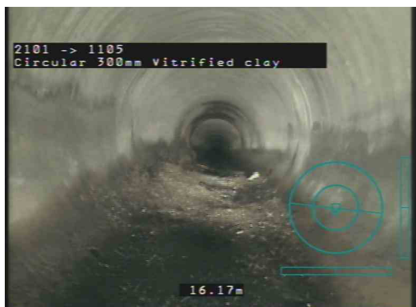
2101X_462ddc81-c59d-43a3-88b2-0b74bcc11d12_20191218_223753_042.jpg, 00:07:54, 16.17 m Roots, mass, 20% cross-sectional area loss, start
