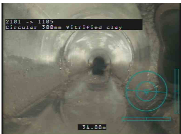
2101X_65f33adf-bb8d-4c29-96e1-156203d14962_20191218_224821_145.jpg, 00:17:51, 34.88 m Settled deposits, fine, 20% cross-sectional area loss, start
