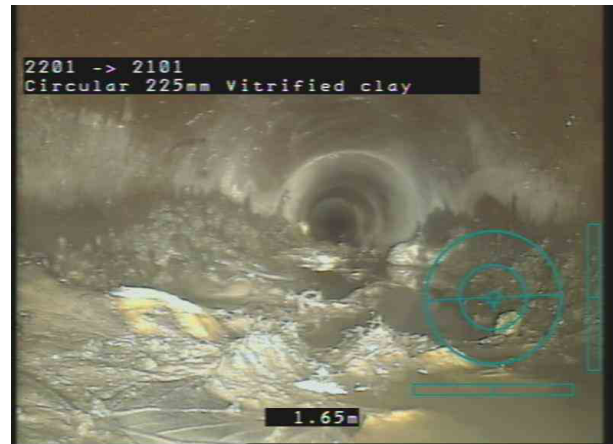
2201X_d7eb6c7f-19ab-49e2-82a2-fbdbc84d65fa_20191219_011003_390.jpg, 00:04:01, 1.65 m Settled deposits, fine, 30% cross-sectional area loss
