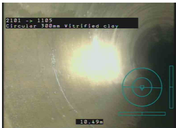
2101X_e43a32e1-e7bb-4540-a1a8-16d7c8271d61_20191218_223652_030.jpg, 00:06:45, 10.49 m Fracture, circumferential from 2 o'clock to 10 o'clock
