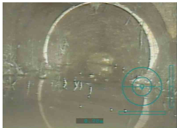
2202X_fa760428-c13d-4e09-a836-50c0f9278e12_20191219_202556_946.jpg, 00:02:29, 0.78 m General remark, blockage visible in distance possible roots
