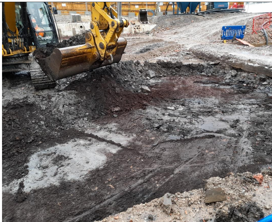
Photo 16: Ground conditions north and north-west of the previously encountered (August 2021) ground contamination. Photograph taken facing the south-east on 20/10/2021.
