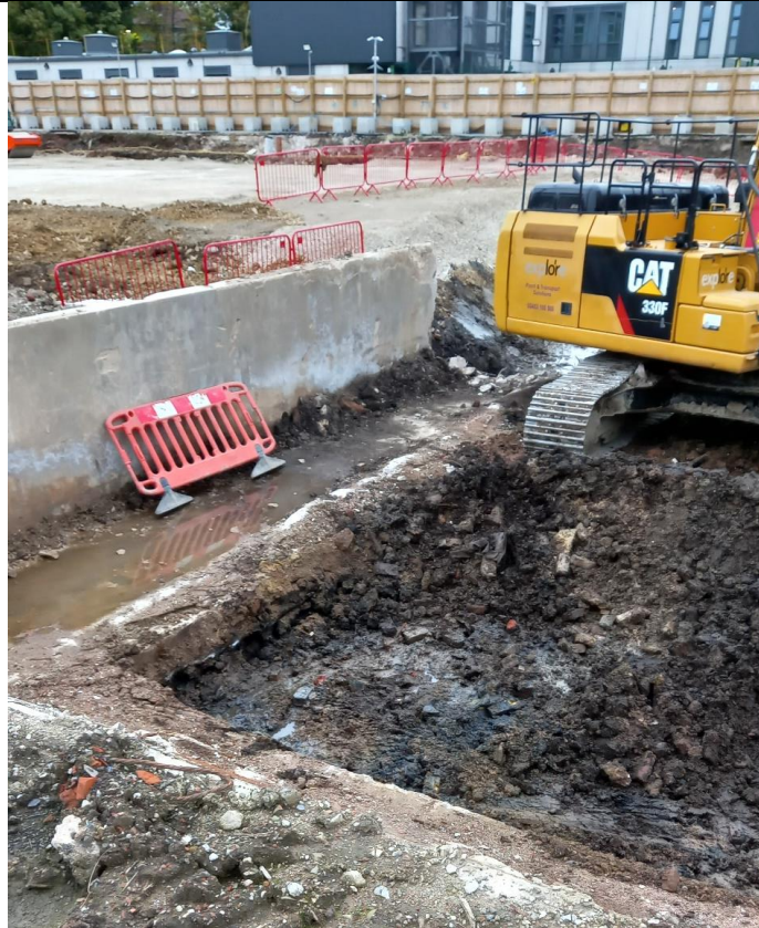
Photo 31: Ground conditions in the south-western corner (Zone E) of the Basement Area; with notable organic / foul odours. Photograph taken facing the north on 27/10/2021.
