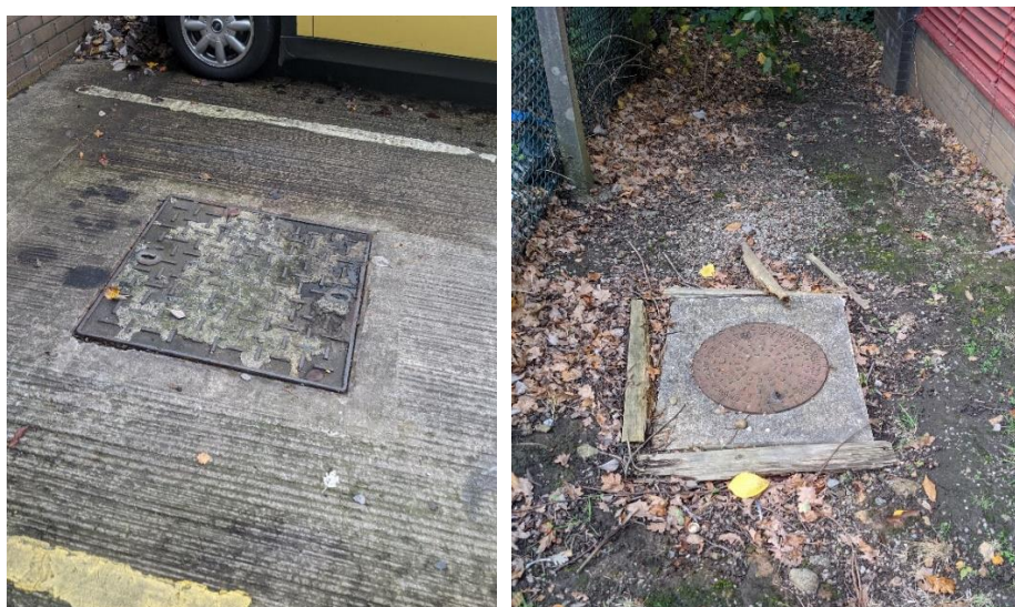
Figure 3: Photograph showing the service access points for water across the site, in the central site section (left) and along the southern boundary (right), with the electricity sub-station visible above the manhole (red).
