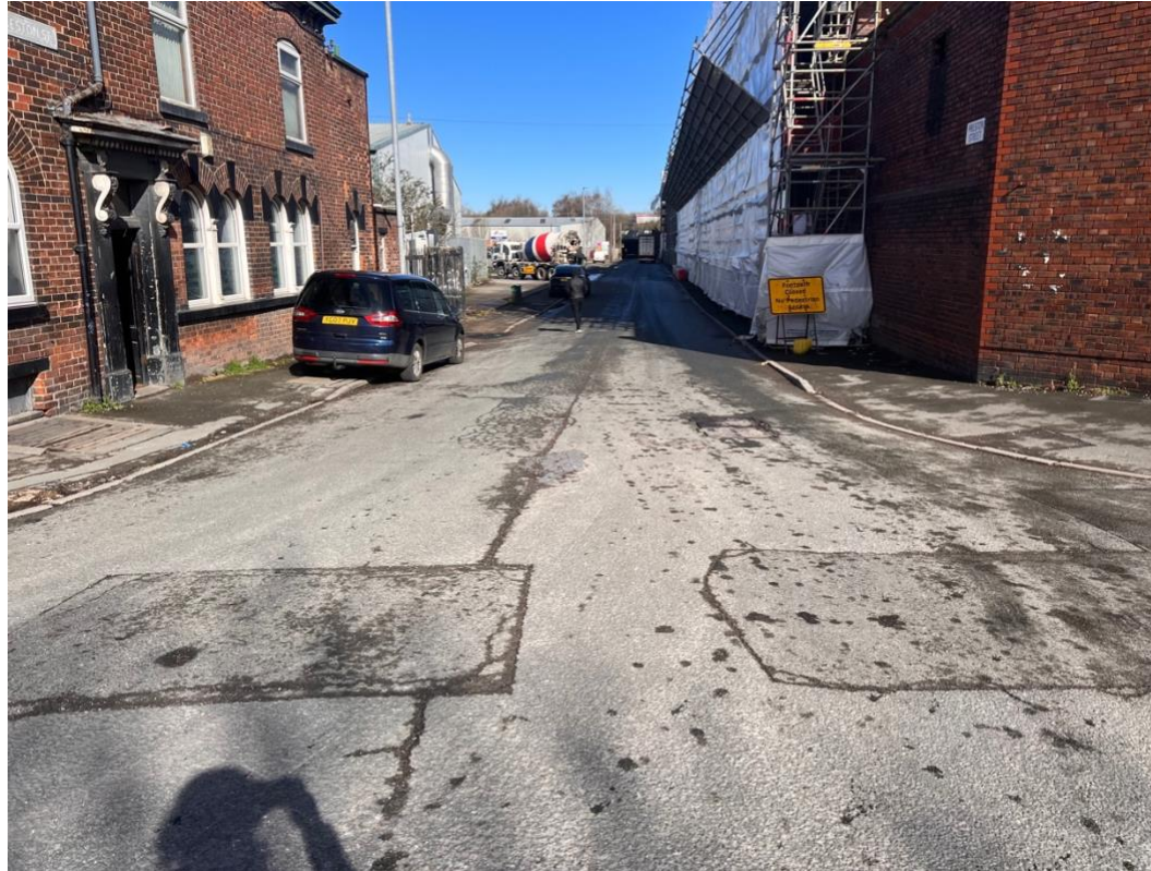
Preston Road at junction with Gorton Lane; Note historic repairs and cracking
