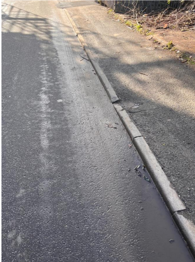
Preston Road; r.h.s. of site entrance (viewed from Preston Rd) Note poor condition of kerbs
