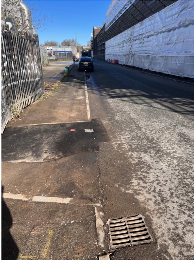
Preston Road outside site entrance; Note poor condition of pavement and historic repairs
