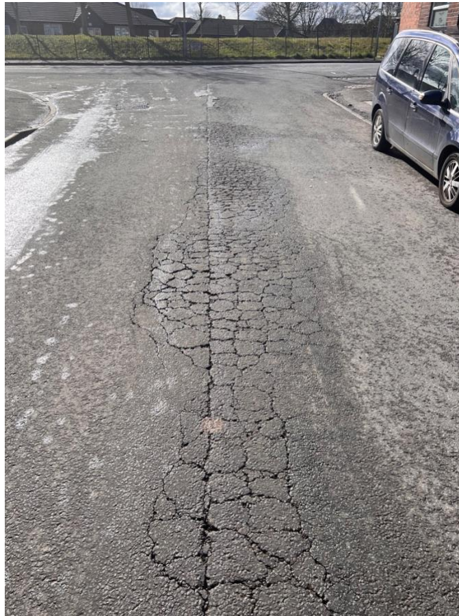
Preston Road towards junction with Gorton Lane; Note the substantial cracking
