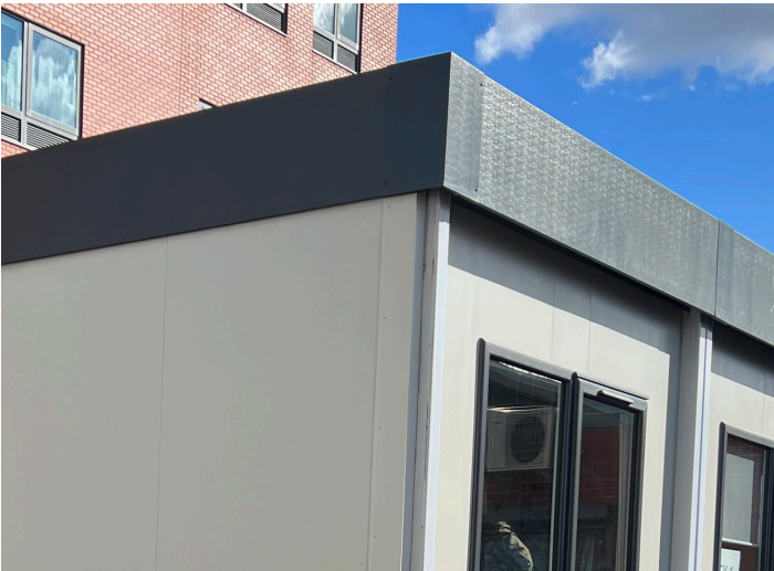
Unit D - Fascia Condition
