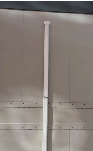
Unit C - Downspout Conditions
