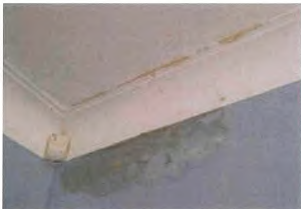
Damage from a leak in a bedroom
